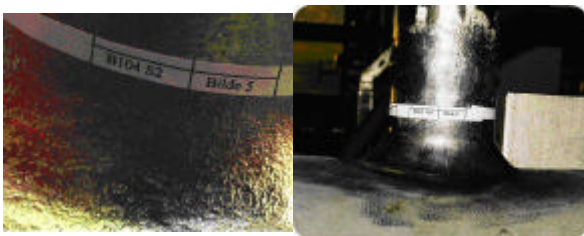
Figure 6 Grinded and needled peened welds from improvements on vibrating gas pipe system
